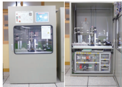
Distribution Panel for the Flow Control EST-0906
