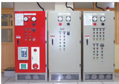
Fire Hydrant / Plumbing / Motor Control Distribution Panel EST-0905
